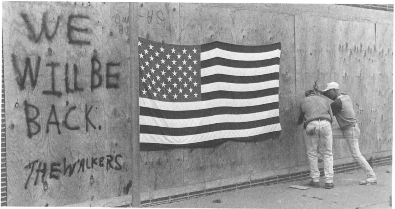
Employees of Walker Stamp and Seal, one of hundreds of damaged businesses near the disaster site in Oklahoma City, board up the shattered exterior of their building. Photo: Carolyn Bauman. Courtesy Fort Worth Star Telegram.
