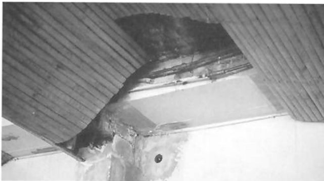
Interior photos show the curved ceiling in the lecture hall, top, and the deterioration.
